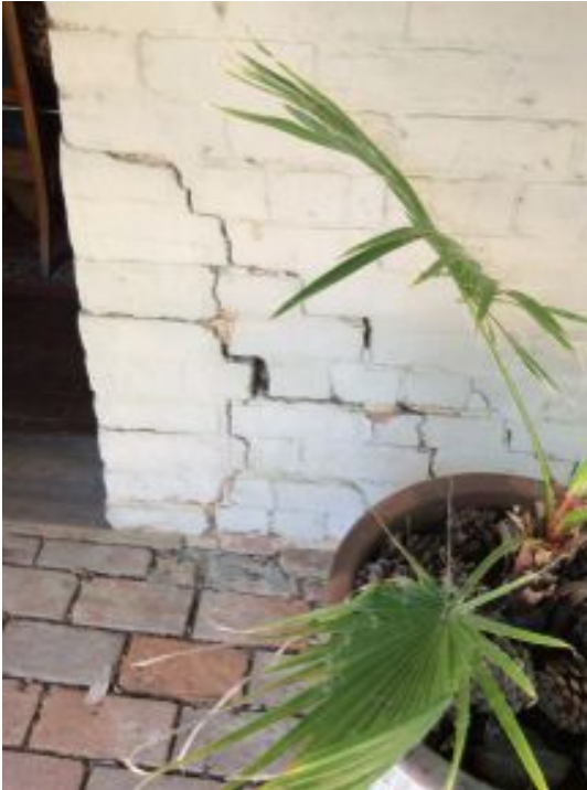
The cracks in the wall
