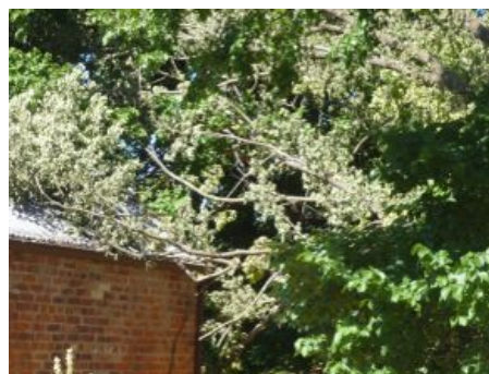
Now the branch rest on the roof of the kitchen outbuilding
